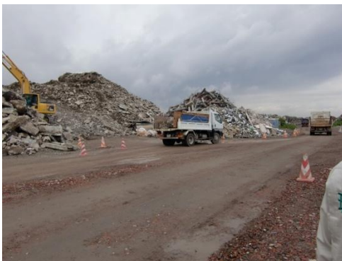
Appropriate separation of disaster waste is important to realize smooth clearing work
